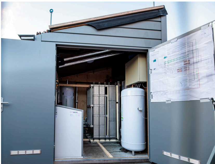
The HEAT-INSYDE system installed in Eindhoven
